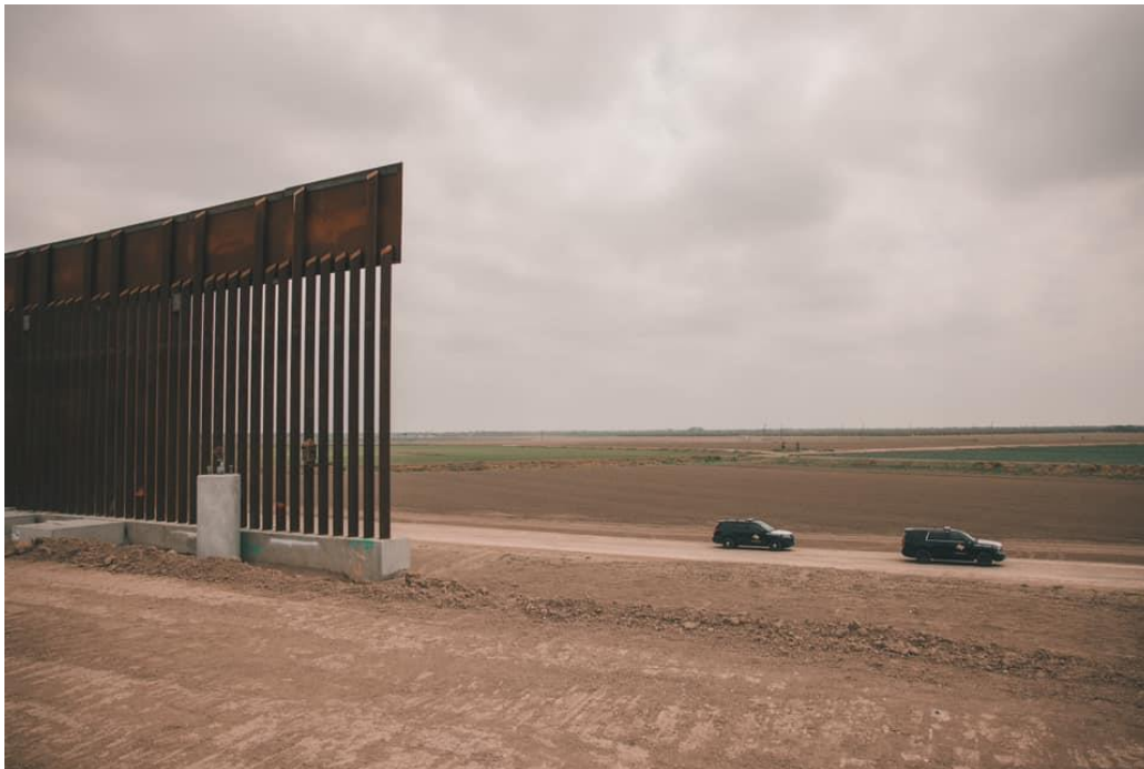
Figure 2. Incomplete Border Wall in the Rio Grande Valley Sector
