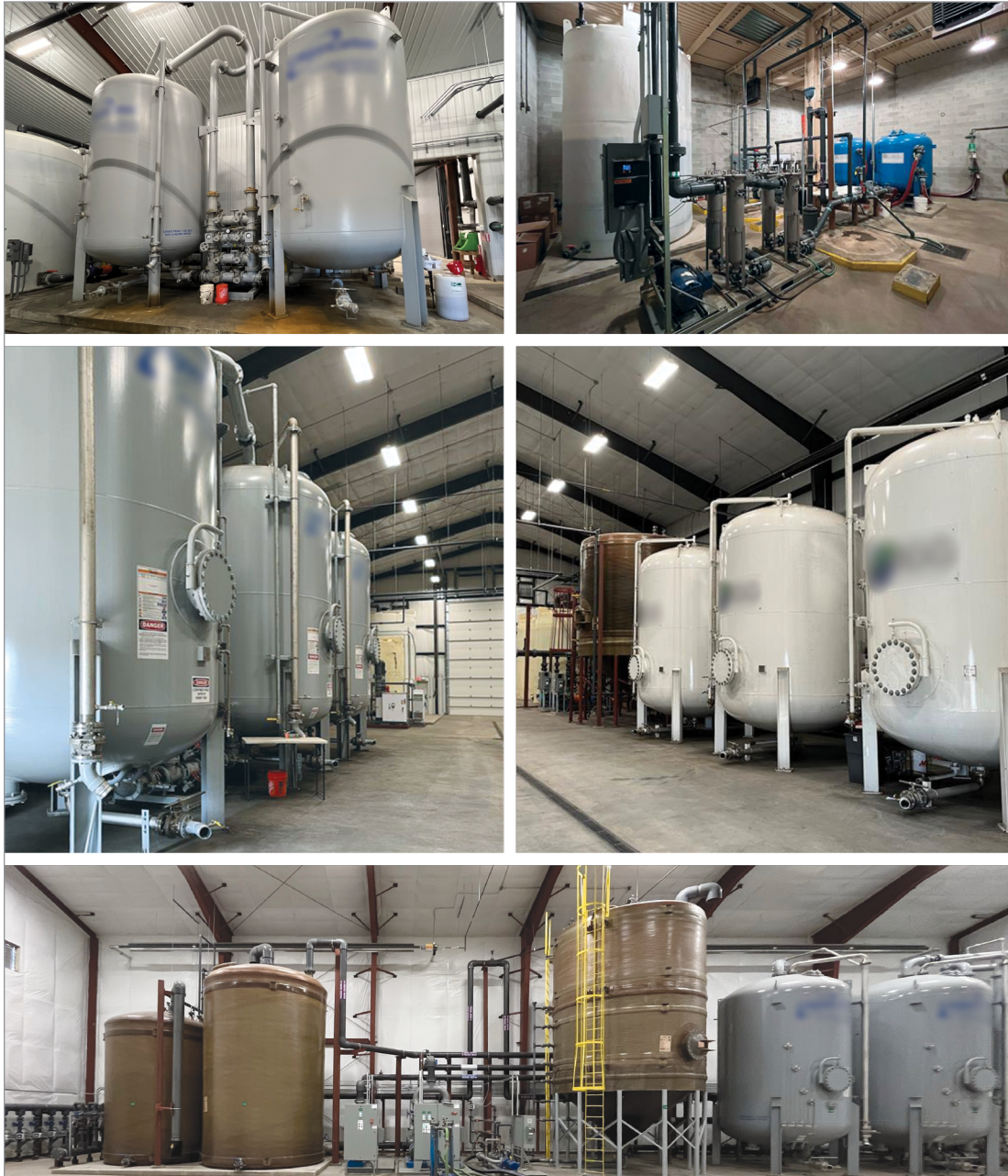
Figure 4. Groundwater Pump-and-Treat Systems at Former Wurtsmith Air Force Base
